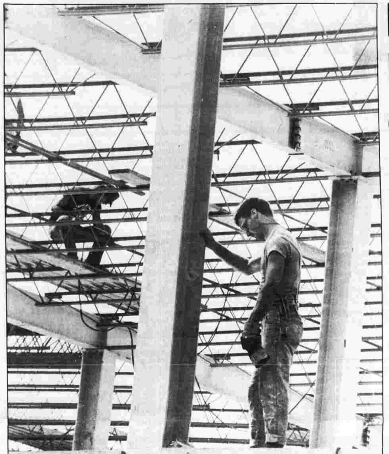
CLOSE INSPECTION - Iron worker Rick Blair of Williamant checks the alignment of an upright beam while a co-worker welds roof beams Monday at the Pavilions at Buckland Hills.
